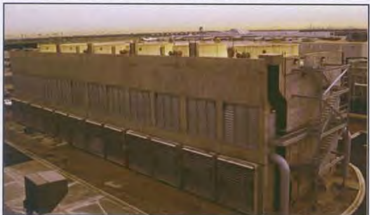
Figure 5. Example of a zero plume tower at a major airport
