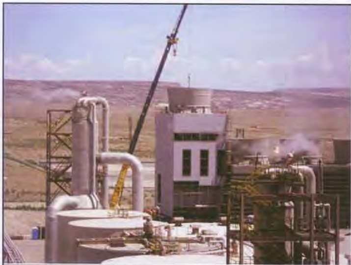
Figure 16. Windows in casing for air supply ducts to modules [photo by Tom Ruisinger]
