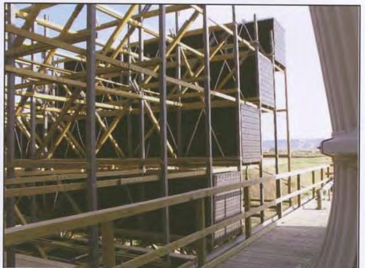
Figure 15. Condensing modules positioned in demonstration cell [photo by Dennis Parker]
